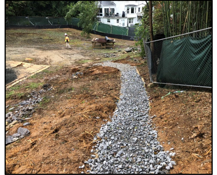
Completed Western Drainage Channel for erosion control and New Super Silt Fence at back
