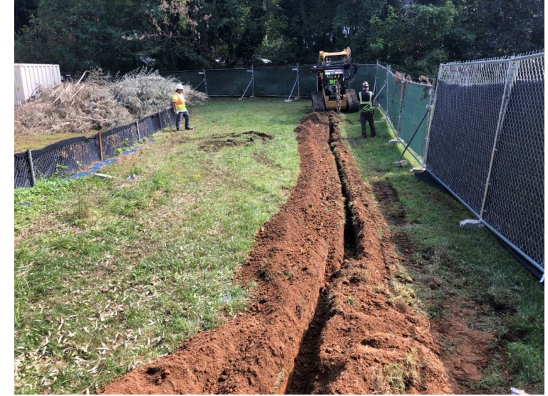
Excavating anchor trench for the Super Silt Fence to be installed within the limit of disturbance along the southwestern edge of the site
