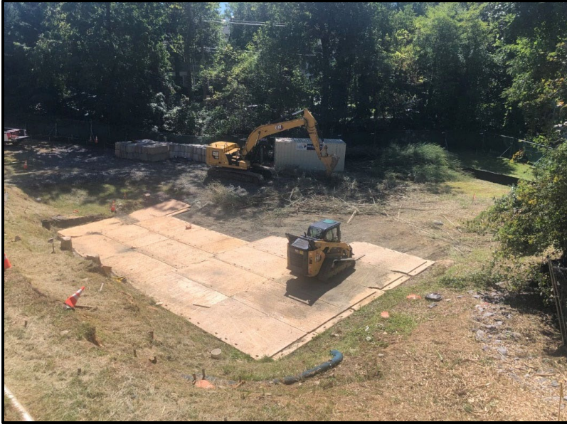
Construction Mats protecting the PSB Foundation Remediation Area and overview of the site
