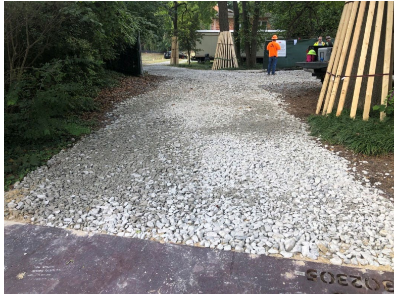
New stone in place for the stabilized construction entrance plus tree protectors installed along the access road
